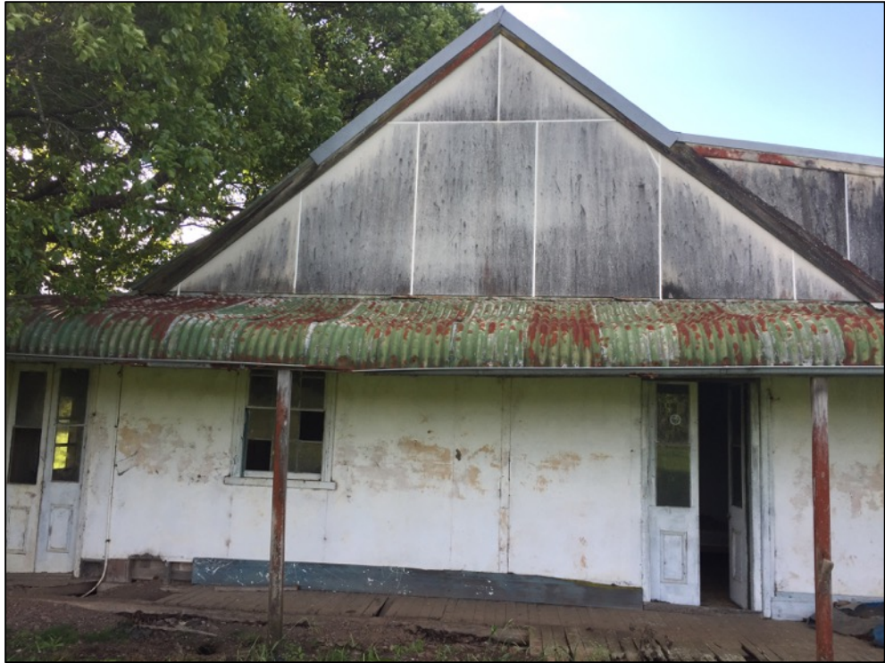
Figure 7: A detail of the dilapidated state of the homestead.
