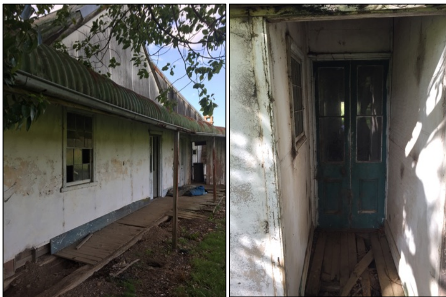
Figures 14 and 15: Exterior photographs of the Old Coomeroo Homestead showing the extent of dilapidation.
