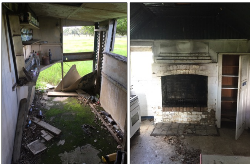
Figure 16 and 17: Internal photographs showing poor condition of the homestead.
